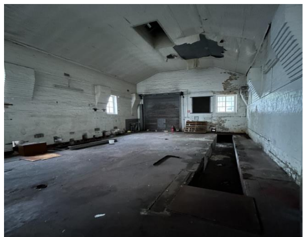
Figure 27 Interior of the substation facing northeast.
